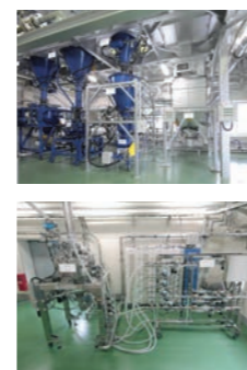
Dust particle handling plant
